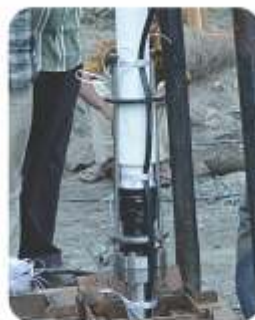
Ensure that pump guard is installed properly
